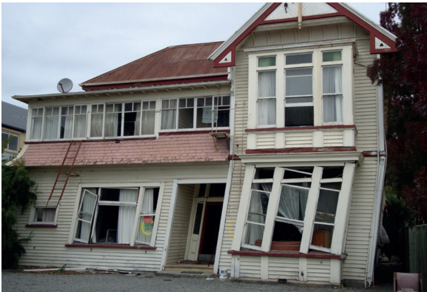
Figure 1. Photo of a residential house from CBD Christchurch, New Zealand (taken by Ihsan E. Bal after 22 February 2011 Christchurch Earthquake M_w 6.2)
